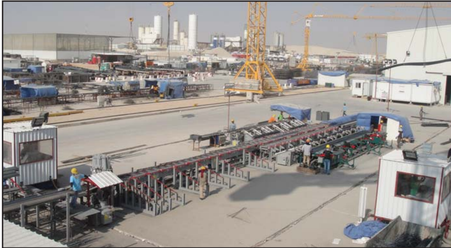
Two KRB Standard Shearlines with bar transfers to double benders operate on the university project site.
