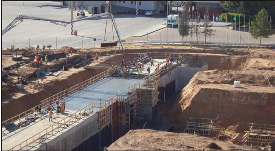
Large amounts of reinforcing steel will go into the two new terminal buildings.
